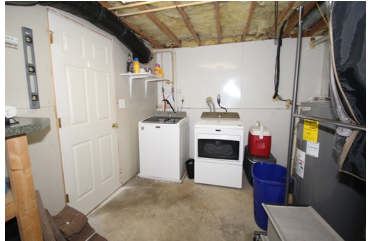
Utility Room in Basement
