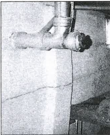
Deflection and cracking such as this in unreinforced concrete block basement walls can now be repaired by a process of placing reinforcement and concrete in the hollow cores of the masonry.
