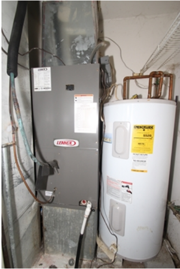
HVAC & Water Heater
