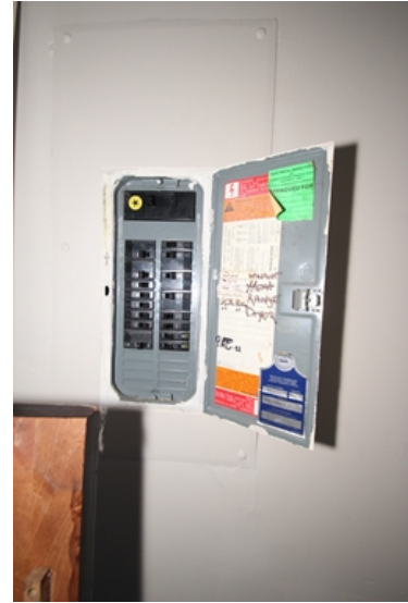
150 amp panel box
